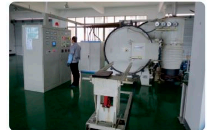
Vacuum brazing furnace
